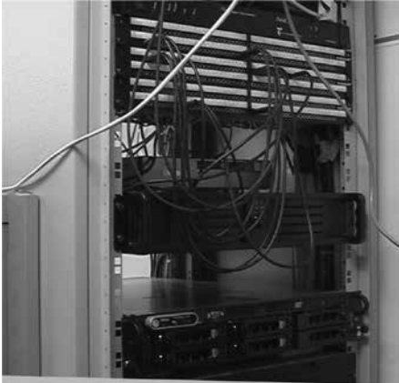
An analog studio—devices are connected with cables.
